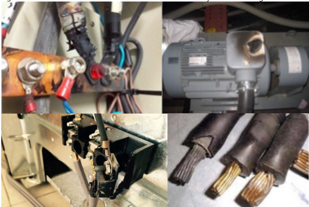
Fig15: Overheated connections due to high resistance
