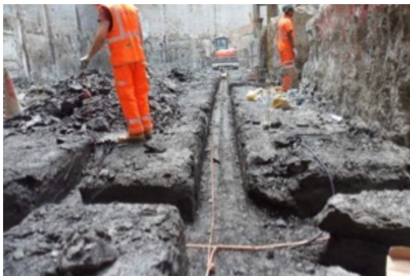
Fig8: Crossrail station earth mat – tested joint resistance before concrete pour (Jonathan King FIET, 2018)
