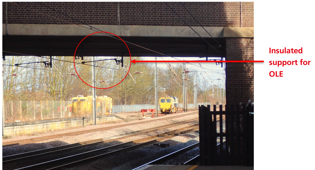
Fig11: OLE running underneath a bridge
