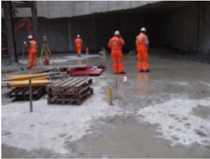
Fig9: Crossrail – concrete poured over earth mat. Has to last at least 120 years (Jonathan King FIET)
