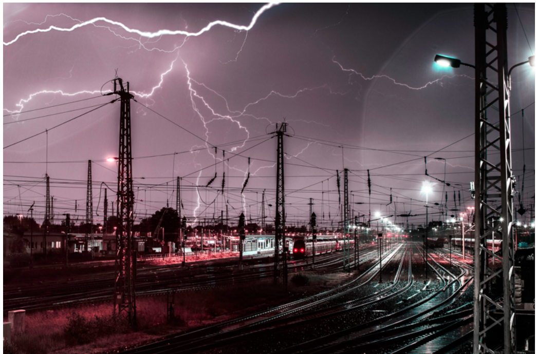
Fig5: Lightning striking overhead line equipment (OLE)
